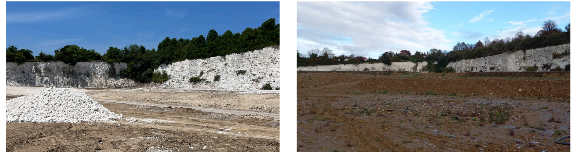
View of site while filling operations were underway (left), and view of completed operations (right).
